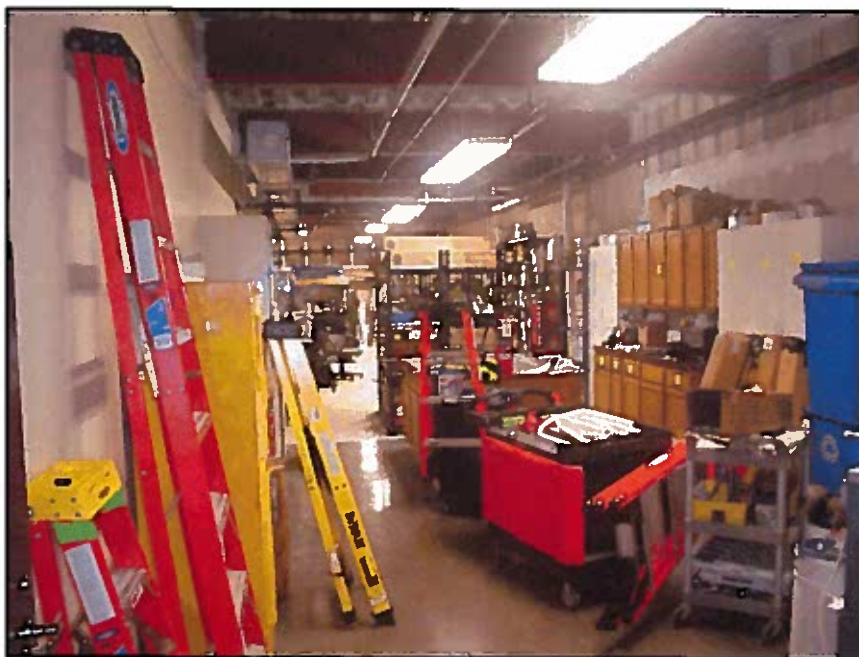
View of the maintenance shop mechanical/storage area on the lower level.
